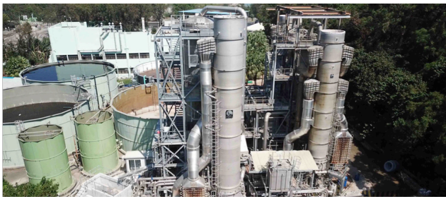
Figure 1. WENT landfill facility – 3300 m 3 /day.
